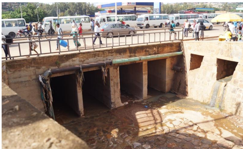
FIGURE 12. NYABUGOGO TRANSPORT HUB BRIDGE ON MPAZI CHANNELIZED RIVER THAT IS PERIODICALLY DAMAGED BY FLUSH FLOODING
